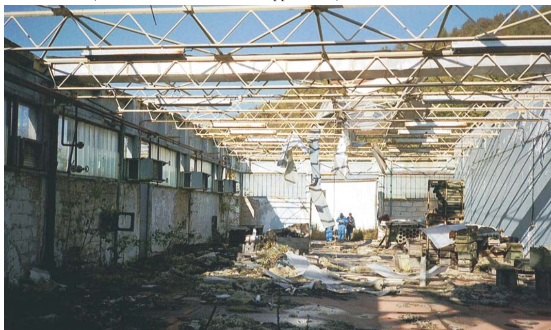
Most buildings were completely destroyed during the attack
